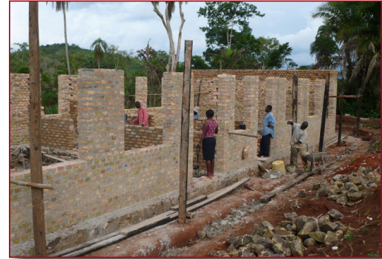
Bricklayers on the orphanage project have made fantastic progress since setting the foundation in August, 2008. The profile of the first building on the campus, the kindergarten classroom, is shown at the top of page, and above.
